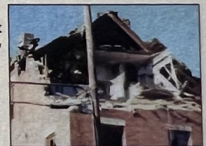
Building demolition revealed the attic space where slaves stayed on their journey to freedom.
